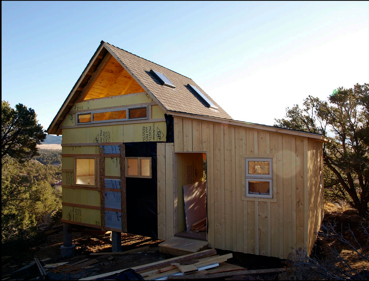
Rough-sawn pine siding goes on over fiberglass-reinforced wallboard and solid styrofoam panels. Most of the windows are home-built.
