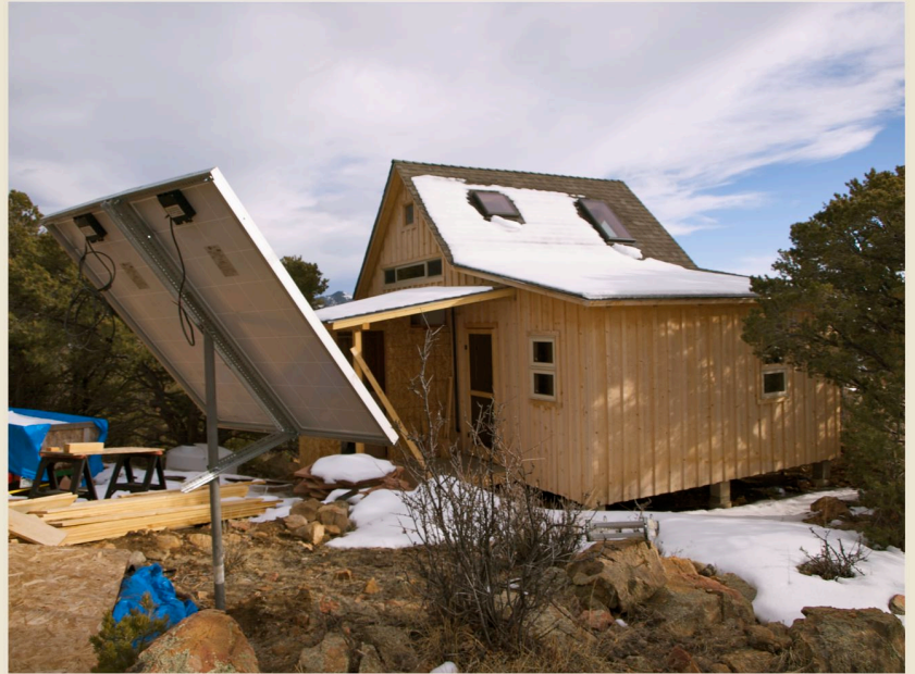
The utility room, which is part of the porch / shower addition, houses batteries for the solar panels (right).
